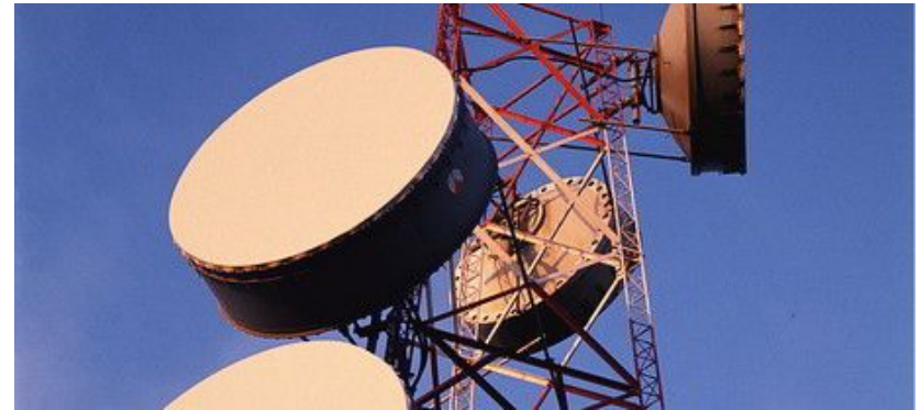
“Microwave” backhaul antennas
